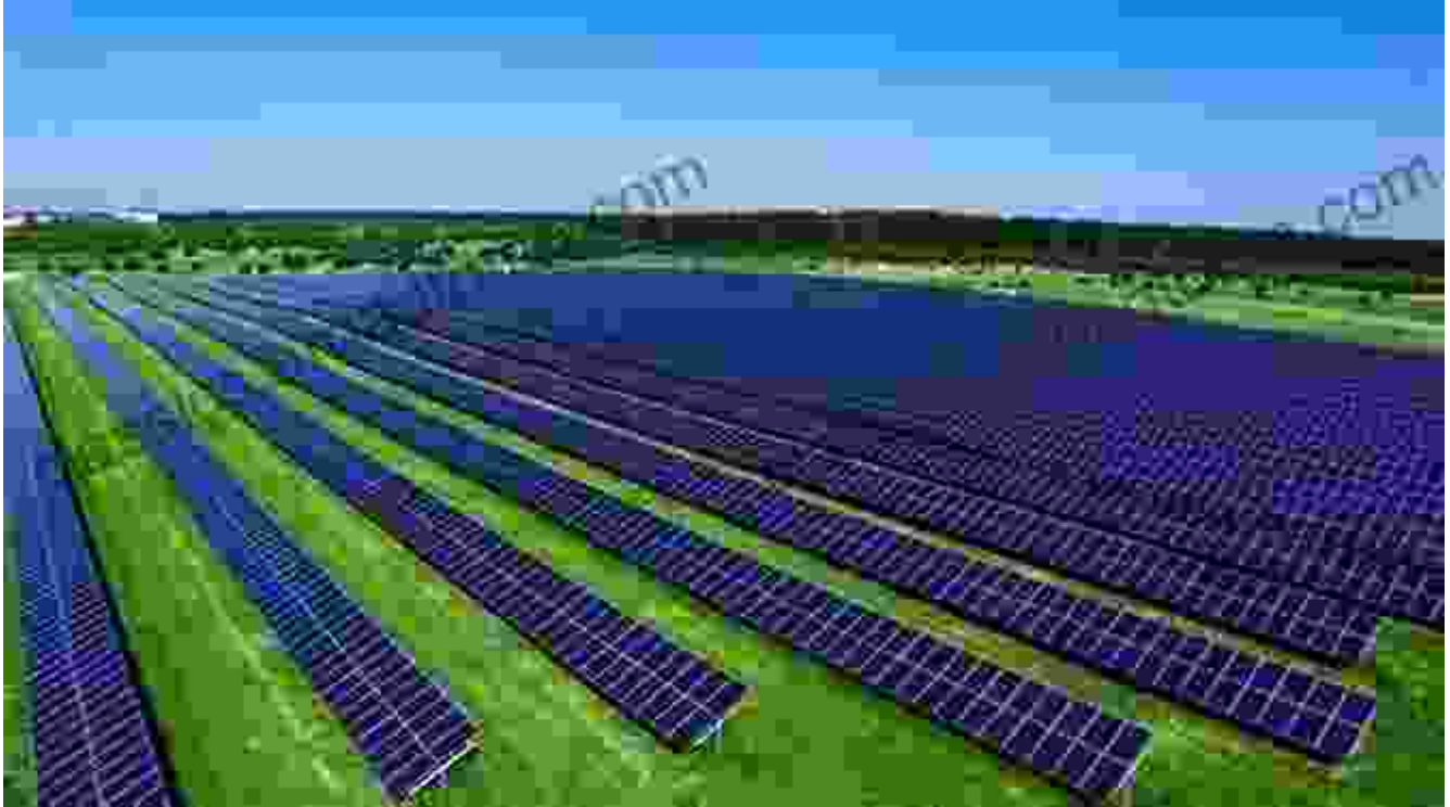
Aerial view of a large-scale photovoltaic array.
